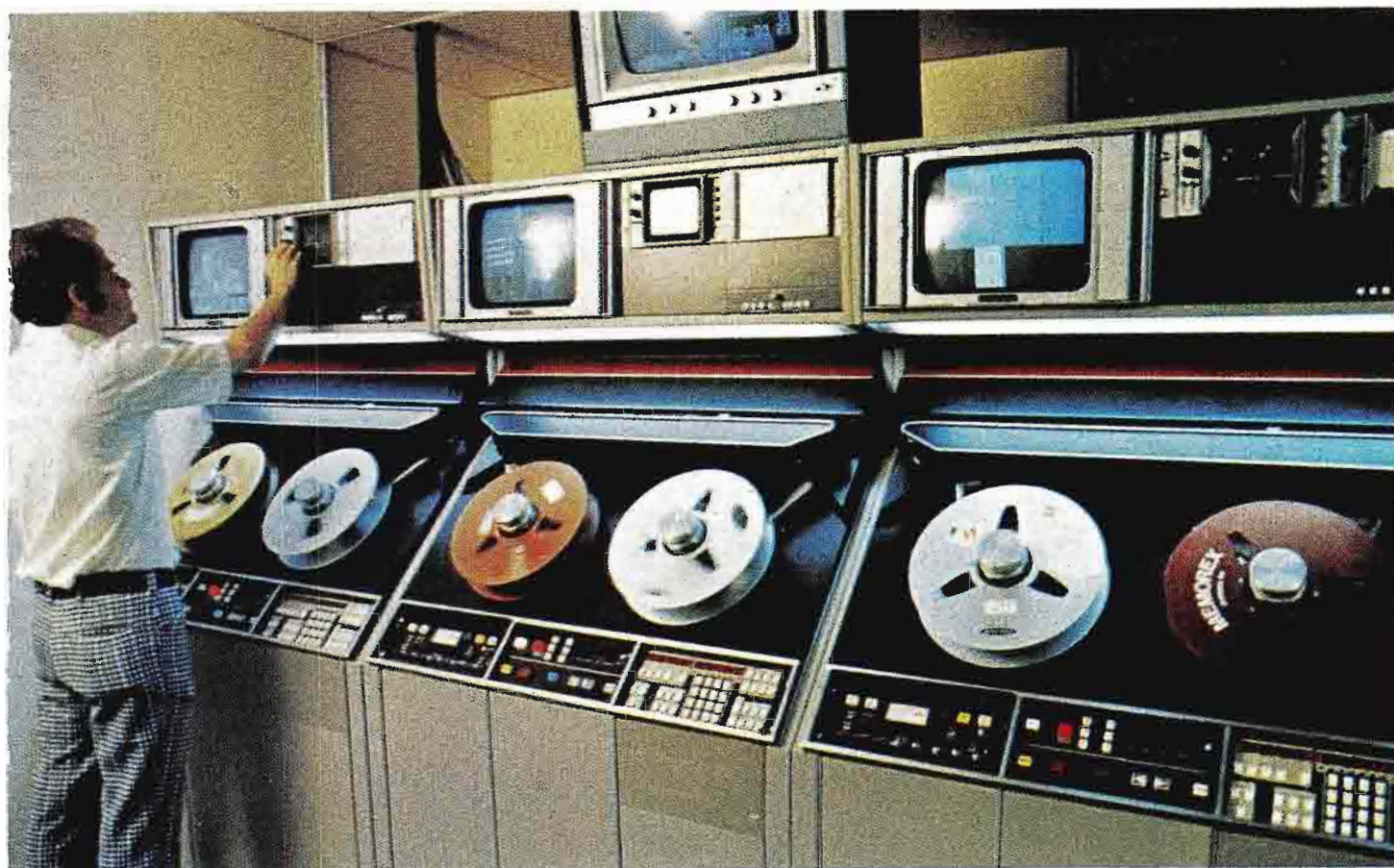
TR-600's are set up for three-machine editing. Both local and remote editing control panels are installed for added flexibility.
